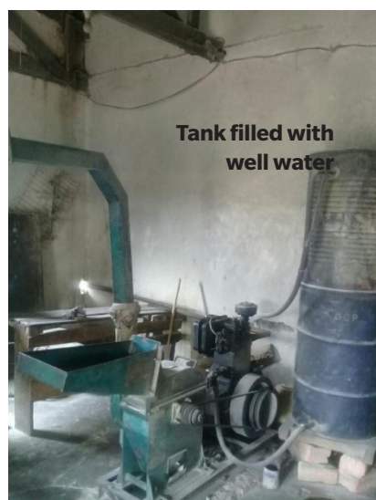
Figure 5: Water cooling modification on diesel mill, source E4I
